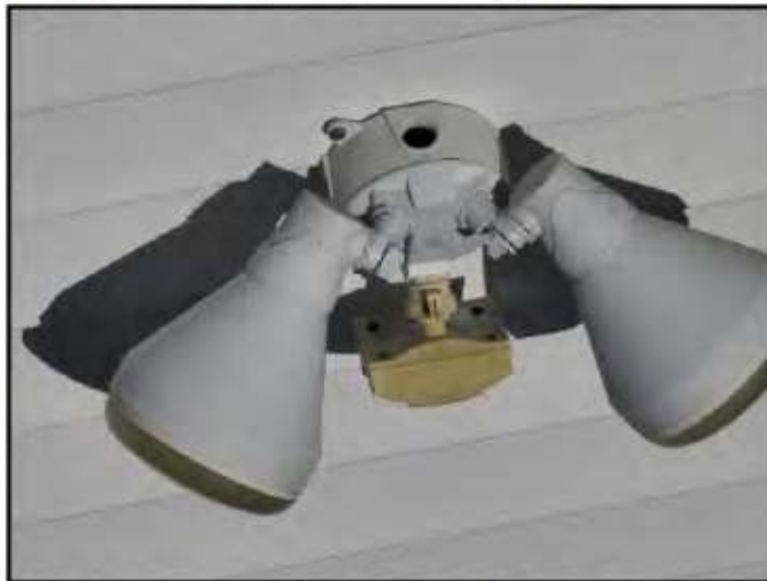
124. Fixtures are missing the matching siding's...
