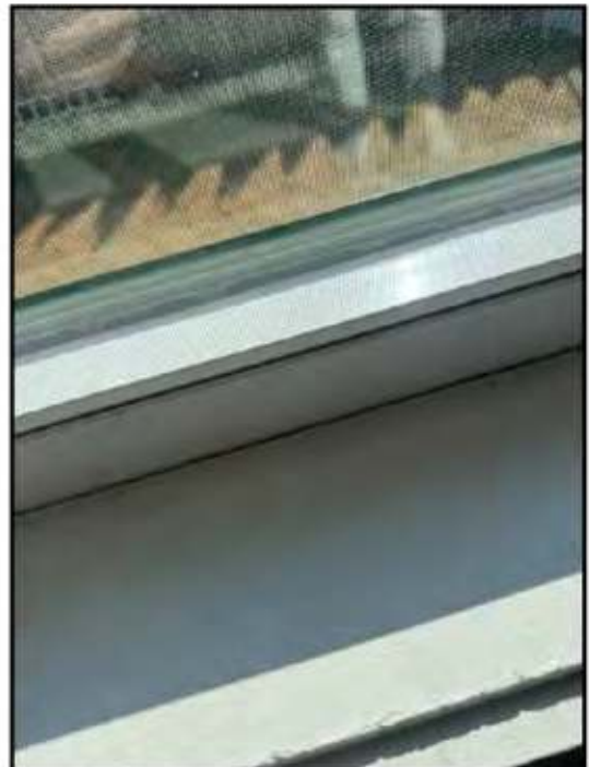
200. Caulking missing, loose or deteriorated
