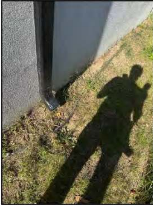
69. Discharge too close to building
