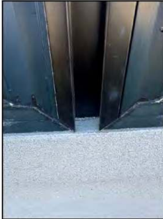
90. Missing or loose pieces
