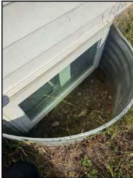
91. Window well cover missing
