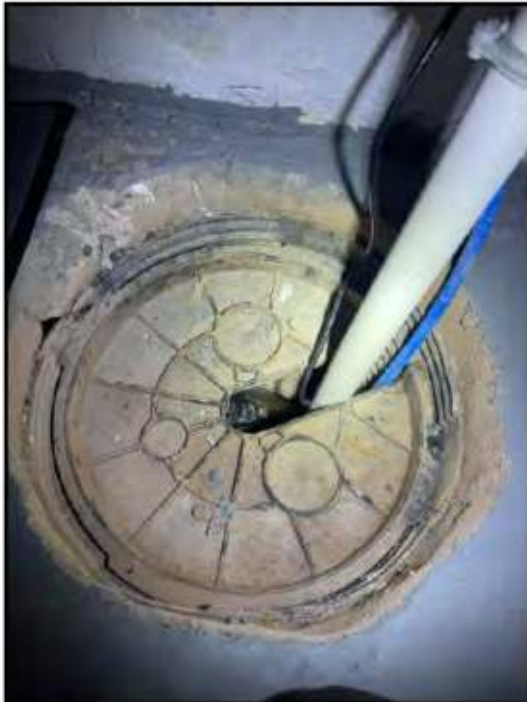
25. Sump pump emergency backup system is highly...
