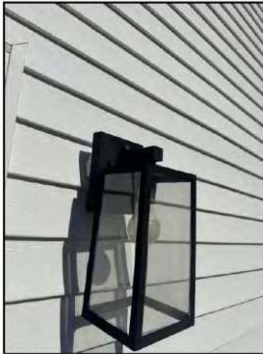
123. Fixtures are missing the matching siding's...
