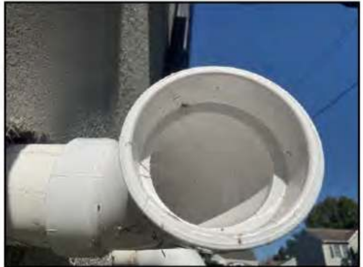
134. Poor vent location, arrangement
