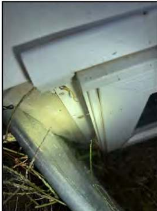
89. Missing or loose pieces
