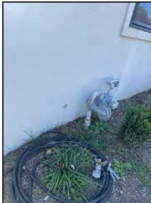
137. Poor vent location, arrangement
