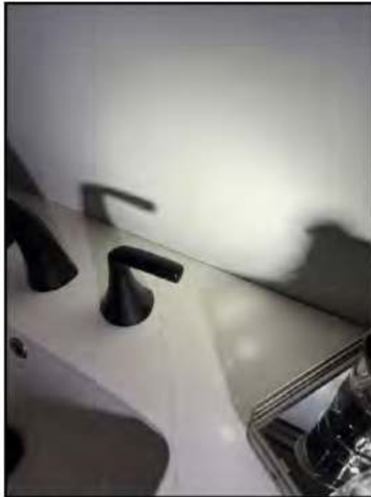
218. Caulking cracked or deteriorating
