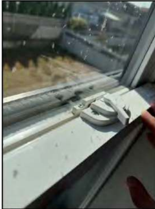
209. Difficult to operate
