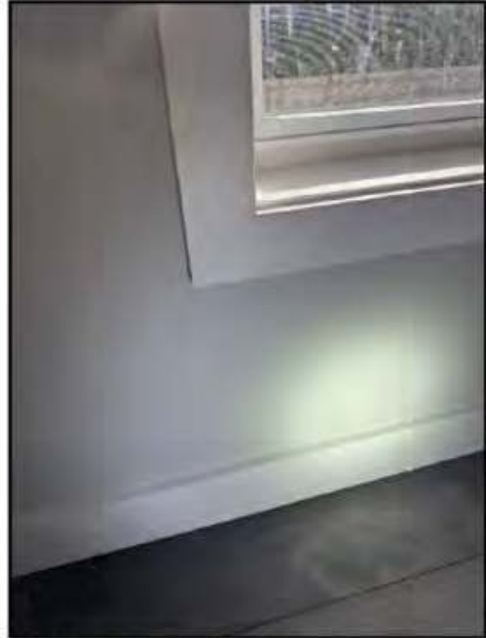
30. Active water leak detected
