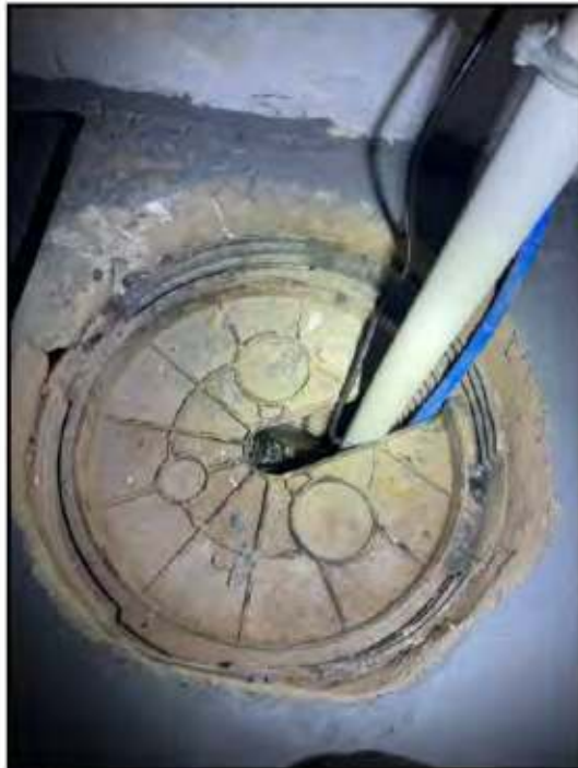
159. Sump pump emergency backup system is highly...
