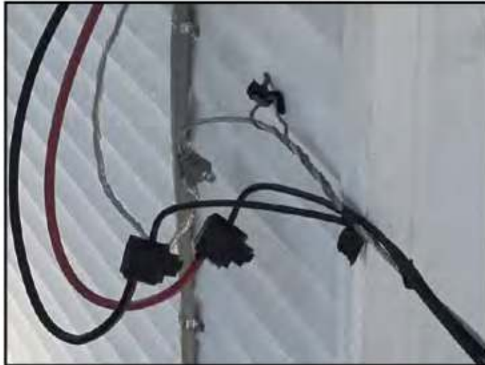
113. Uninsulated Service Entrance wire holder
