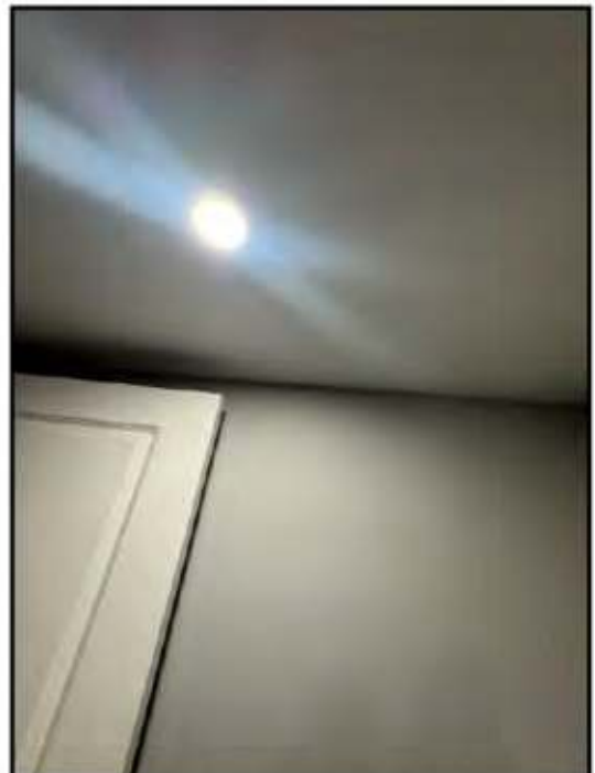
34. Active water leak detected
