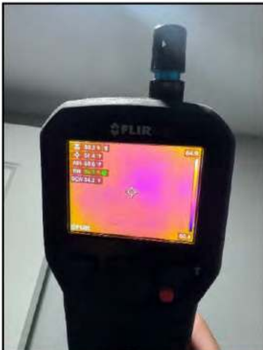
33. Active water leak detected
