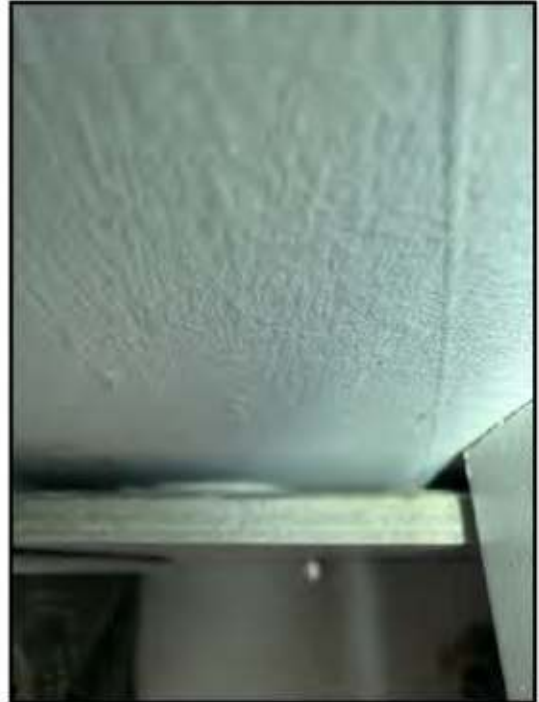
189. Poor installation of tiled backsplash
