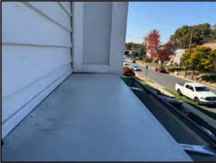
9. Possible water infiltration behind EIFS
