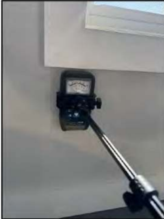
29. Active water leak detected
