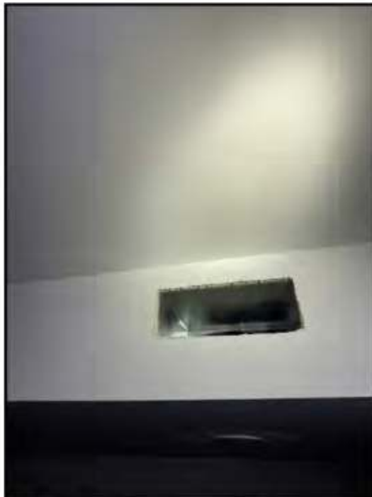
147. Supply register/diffuser is missing
