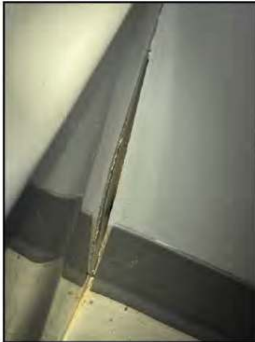
166. Caulking loose, missing or deteriorated
