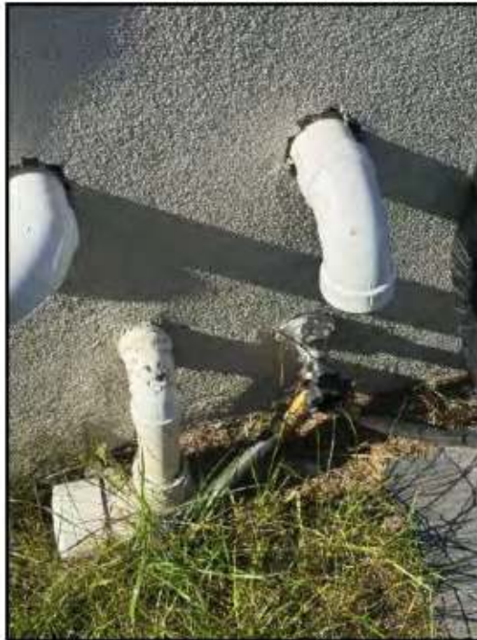
20. Sump pump discharge point was not found at...
