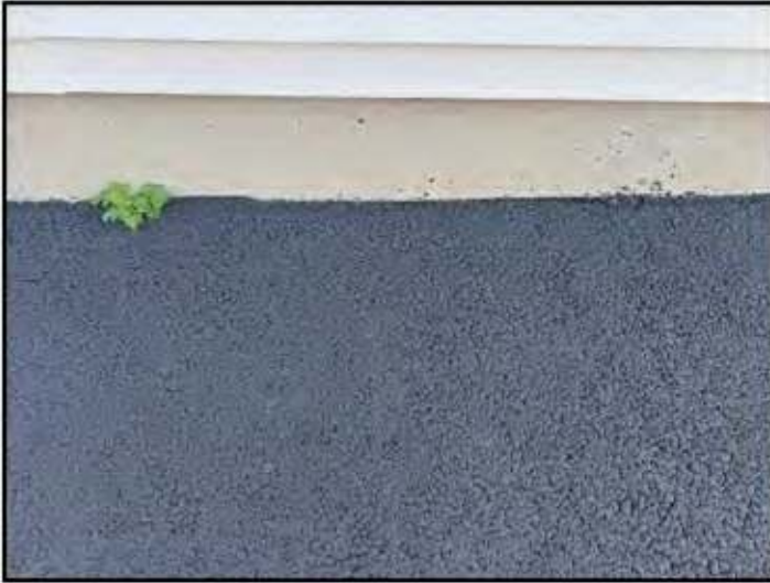
102. Improper slope or drainage
