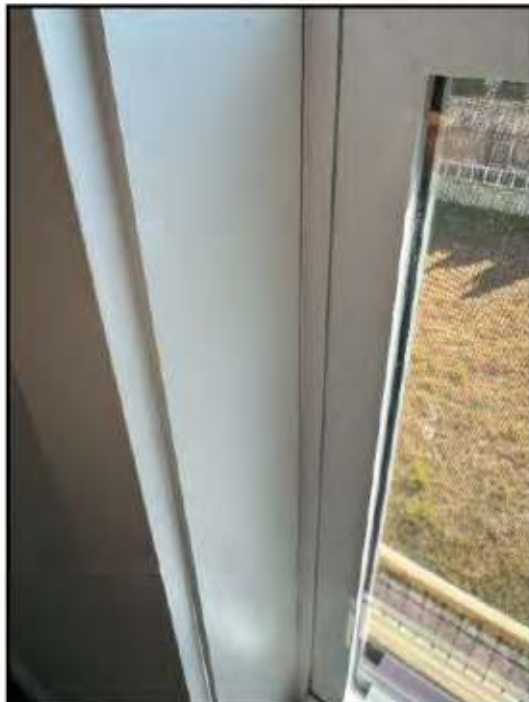
199. Caulking missing, loose or deteriorated
