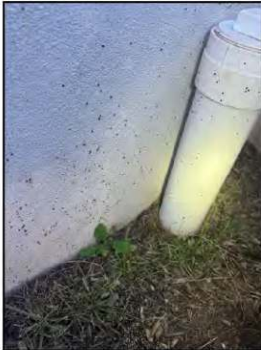
11. Possible water infiltration behind EIFS
