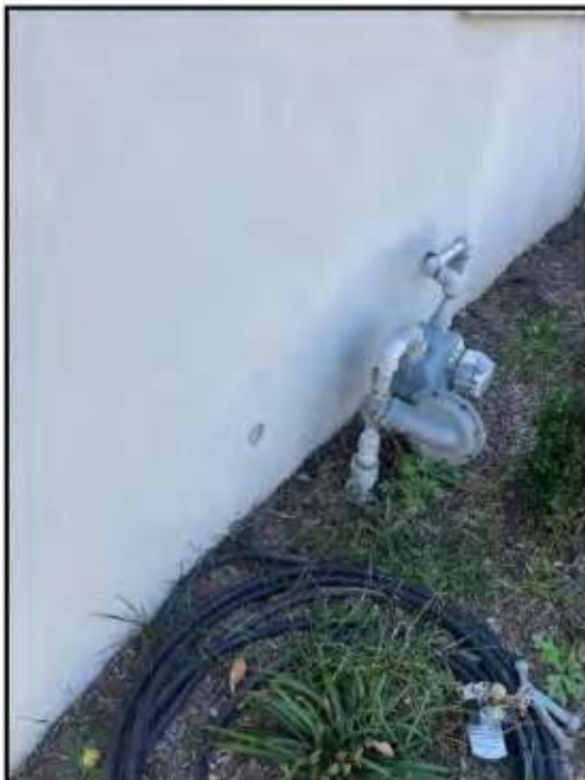
14. Poor vent location, arrangement
