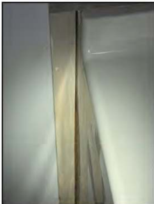
27. Tile loose, broken or missing
