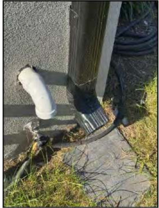
70. Discharge too close to building
