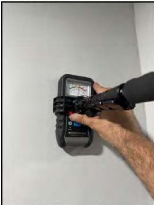
183. Active water leak detected
