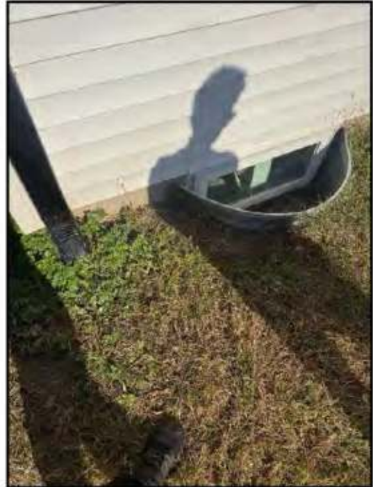
103. Improper slope or drainage
