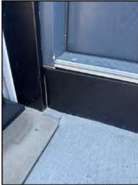
93. Poor support under threshold
