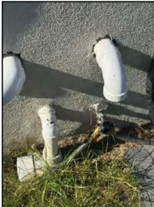
154. Sump pump discharge point was not found at...
