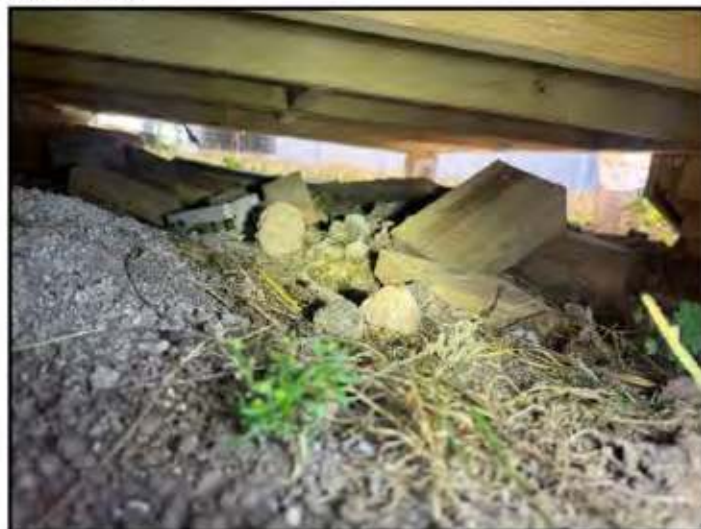
107. Construction debris seen under deck
