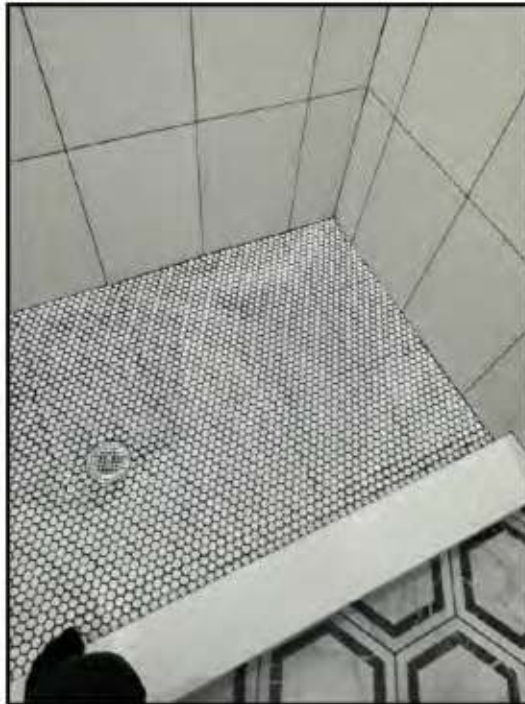
176. Grout sealant recommended
