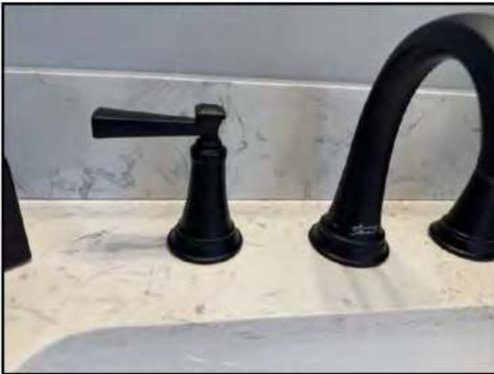
216. Caulking cracked or deteriorating
