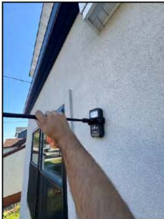
7. Possible water infiltration behind EIFS
