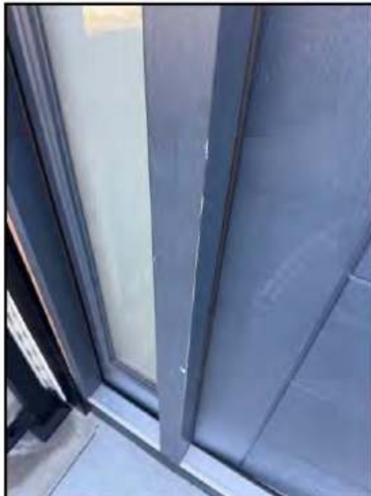
92. Paint or stain needed
