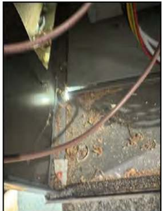
132. Air leakage entering from return side
