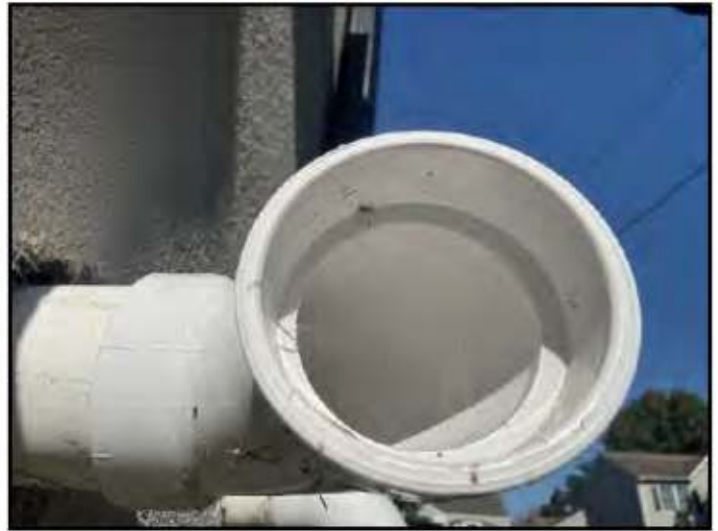
13. Poor vent location, arrangement
