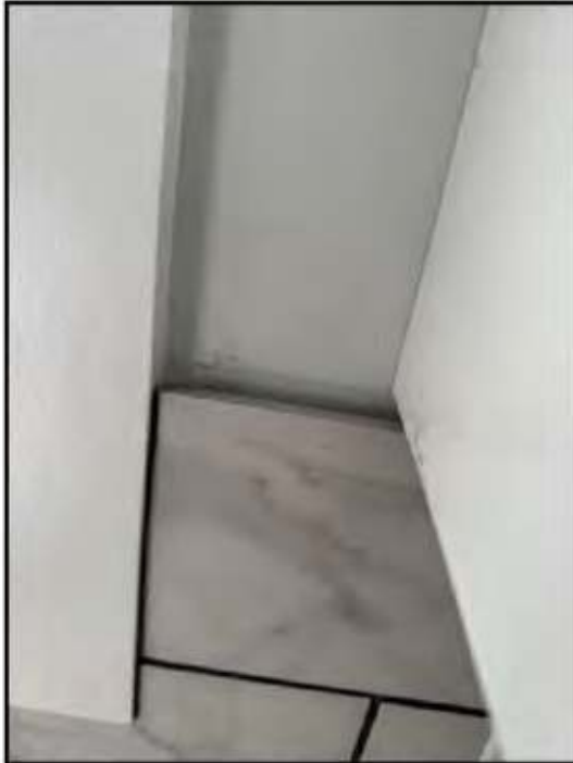
188. Poor installation of tiled backsplash
