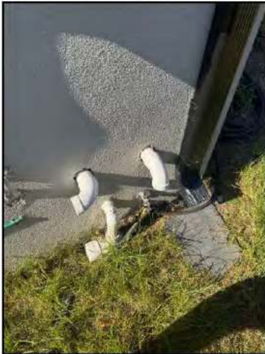
12. Poor vent location, arrangement
