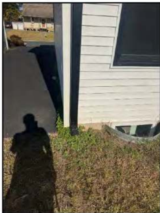
67. Discharge too close to building
