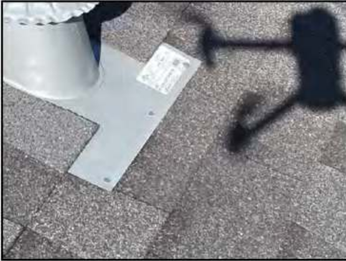
65. Fasteners - exposed / missing
