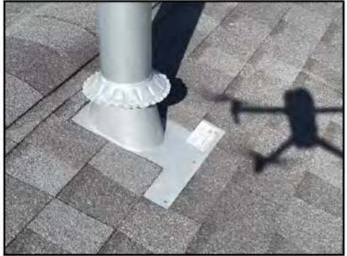
66. Fasteners - exposed / missing
