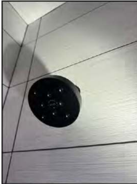
175. Loose shower head
