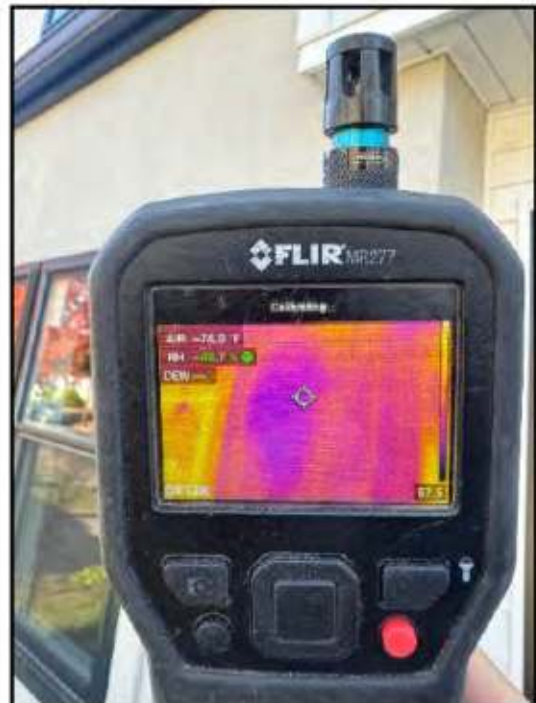
8. Possible water infiltration behind EIFS
