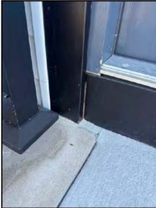
94. Damaged, cracked or loose
