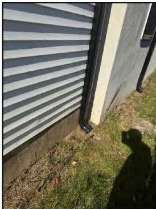
68. Discharge too close to building
