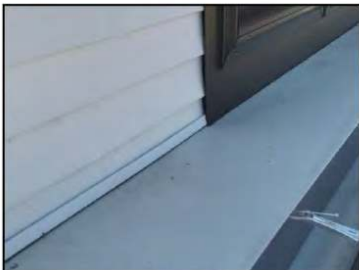
80. Possible water infiltration behind EIFS
