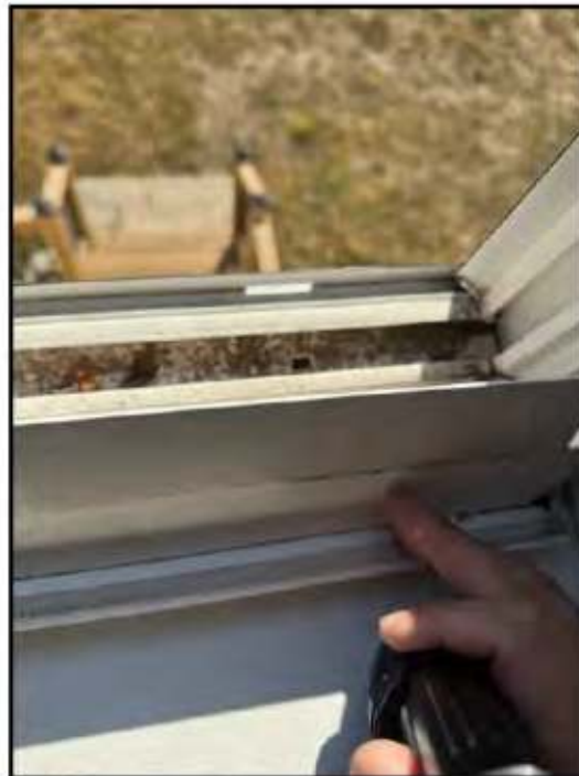
208. Sash coming apart
