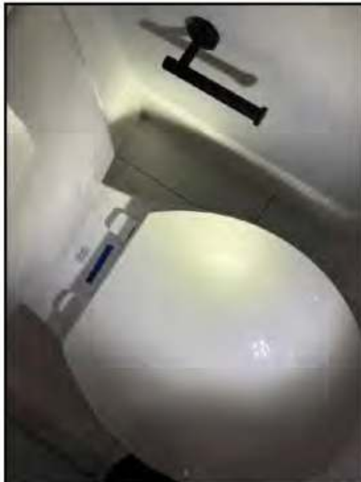
177. Damaged toilet seat
