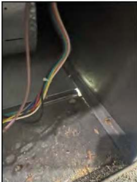
131. Air leakage entering from return side
