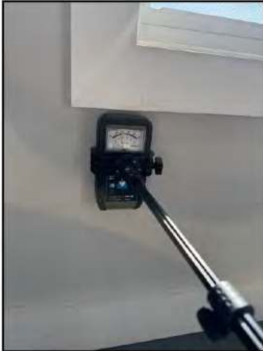
181. Active water leak detected
