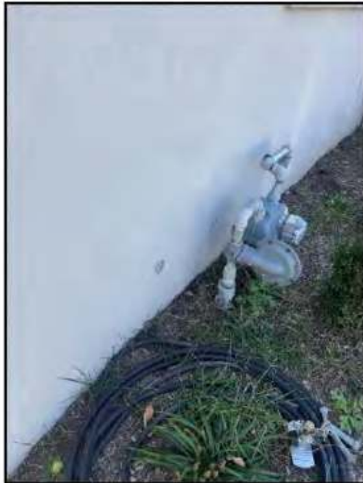
135. Poor vent location, arrangement
