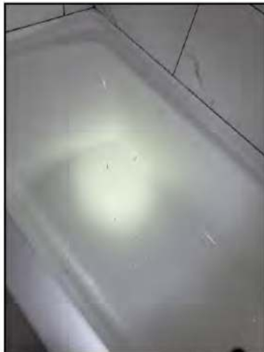
168. Grout loose, missing or deteriorated
