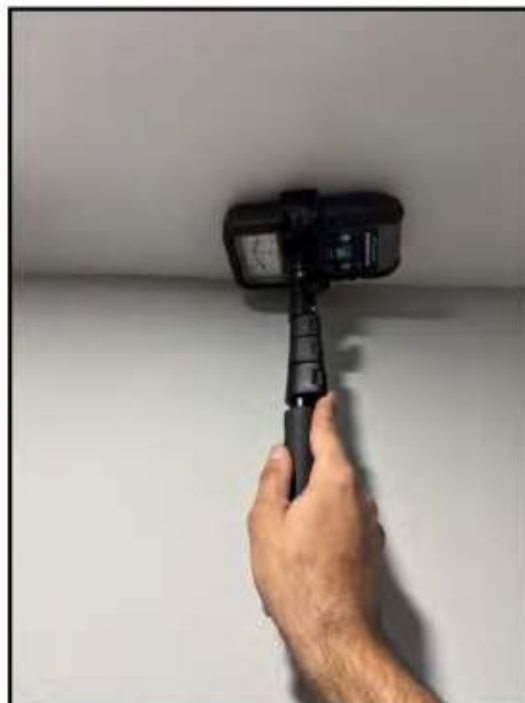
187. Active water leak detected
