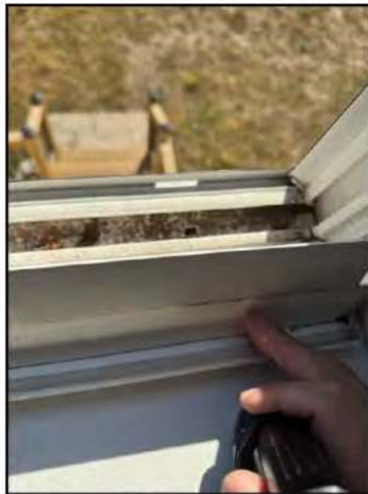
36. Sash coming apart
