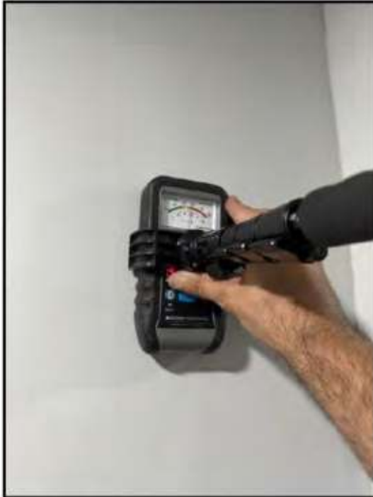
31. Active water leak detected
