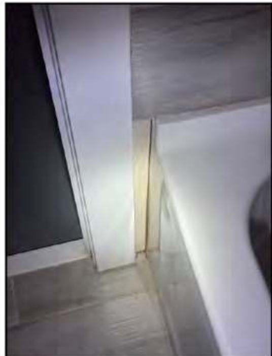
170. Tile loose, broken or missing
