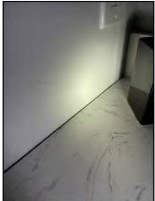
217. Caulking cracked or deteriorating
