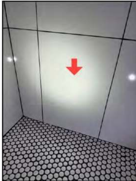
173. Tiles, loose, cracked or broken
