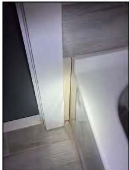
28. Tile loose, broken or missing
