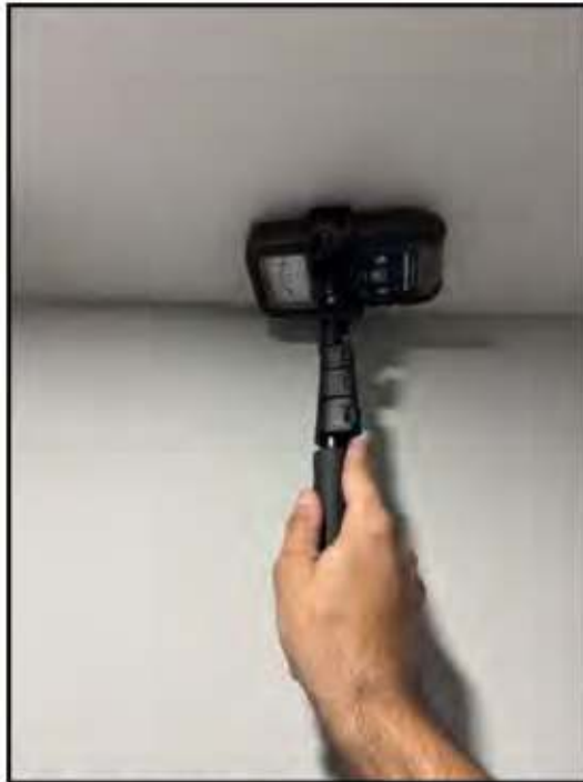
35. Active water leak detected
