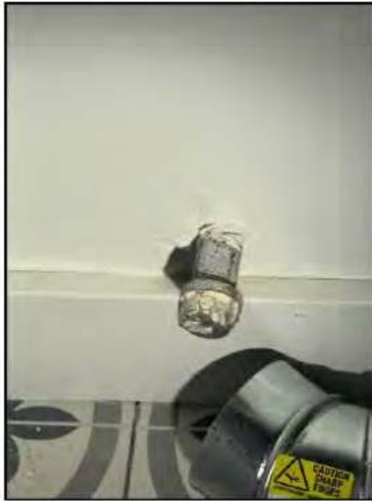
19. Missing shut off valve
