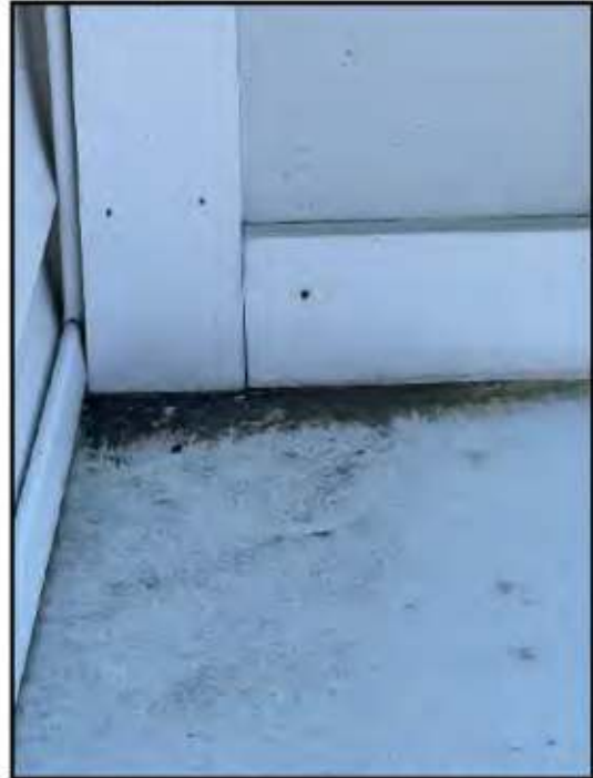
10. Possible water infiltration behind EIFS
