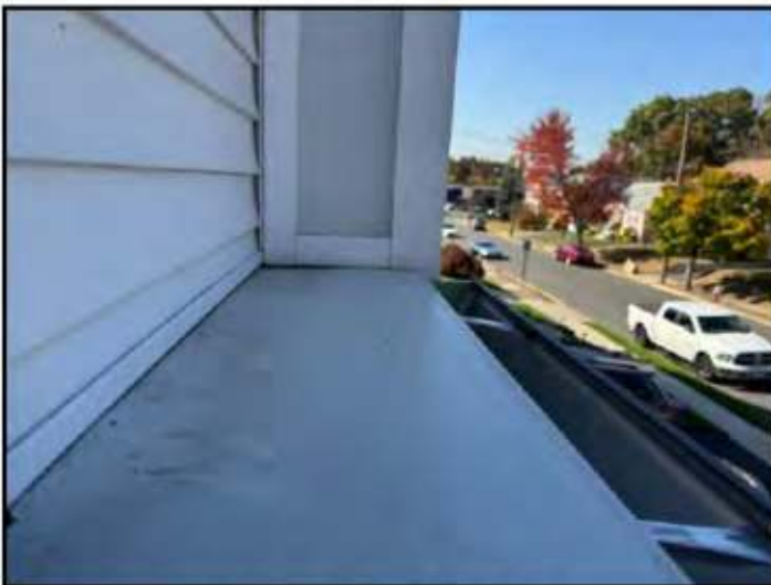
85. Possible water infiltration behind EIFS
