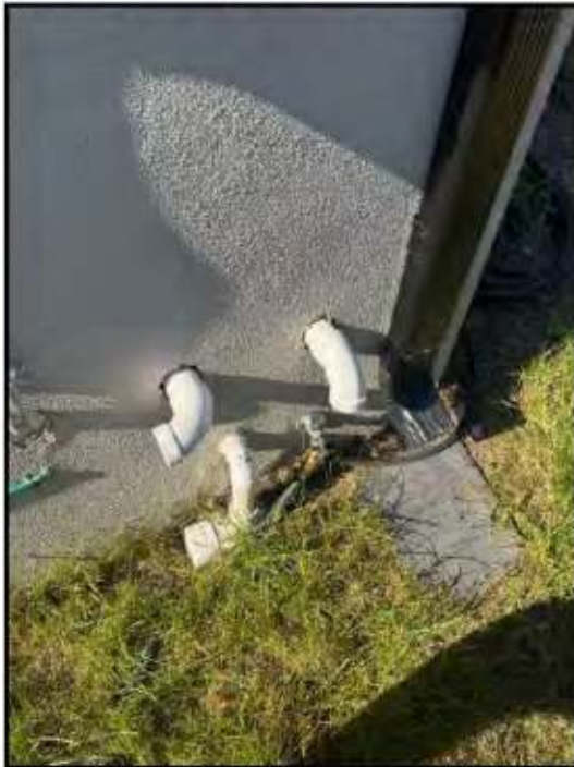
133. Poor vent location, arrangement
