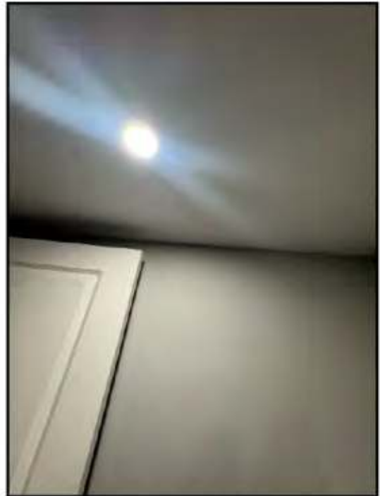
186. Active water leak detected
