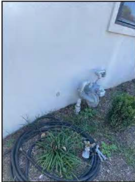
16. Poor vent location, arrangement
