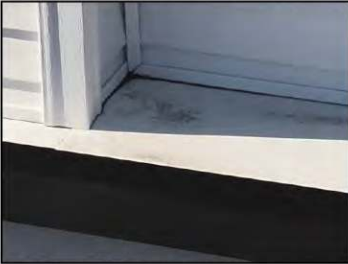
1. Possible water infiltration behind EIFS
