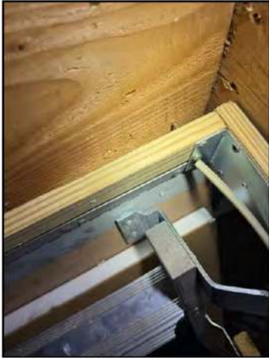
149. Not well secured
