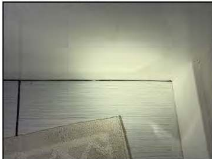
167. Caulking loose, missing or deteriorated
