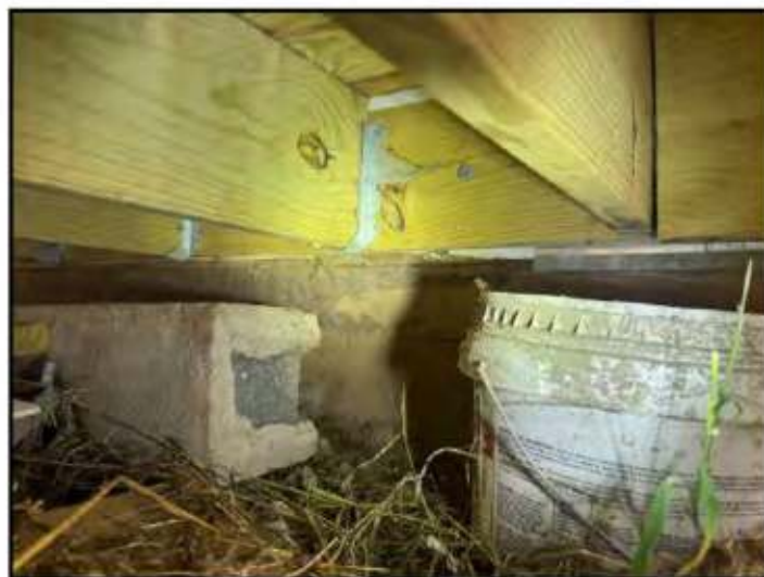
98. Missing flashing at deck connection
