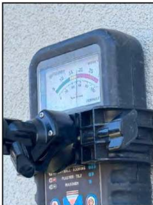
82. Possible water infiltration behind EIFS
