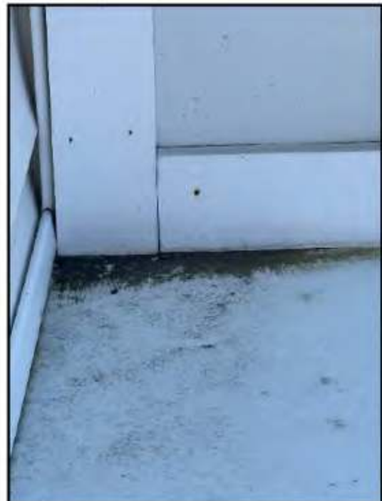
86. Possible water infiltration behind EIFS
