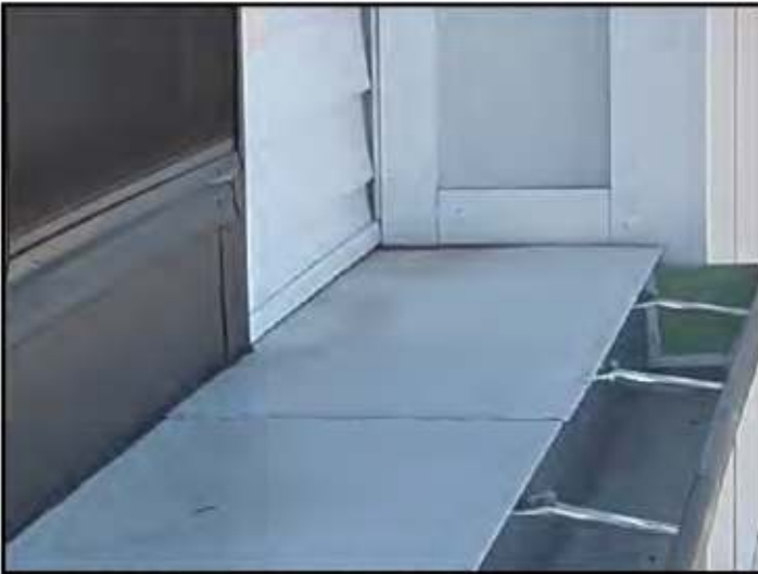
3. Possible water infiltration behind EIFS
