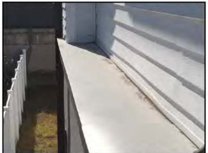
78. Possible water infiltration behind EIFS
