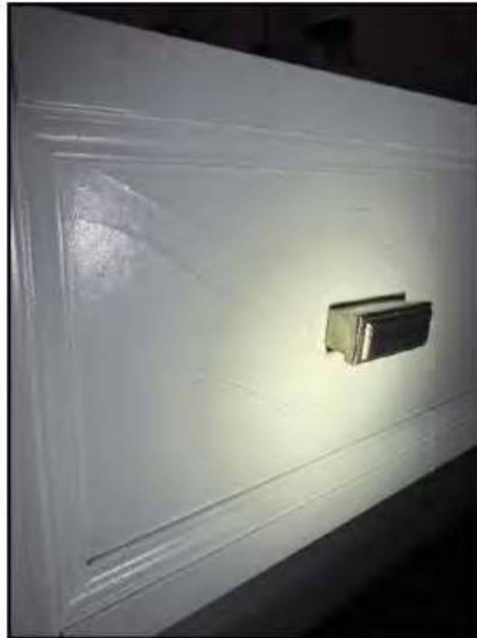
213. Stained, worn, damaged
