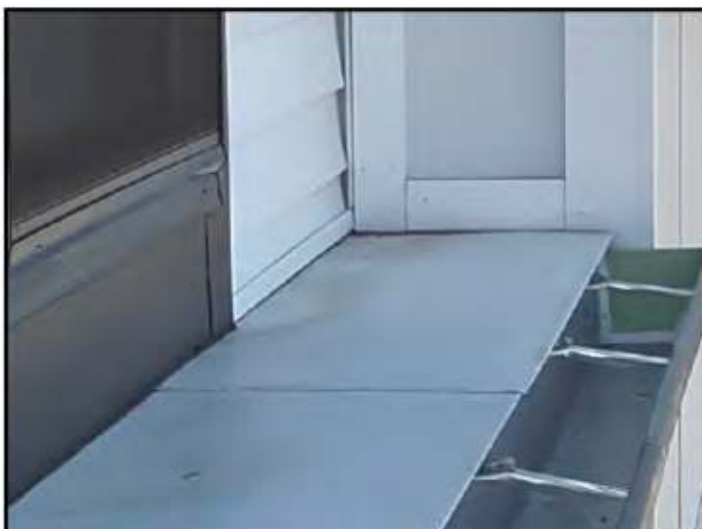
79. Possible water infiltration behind EIFS
