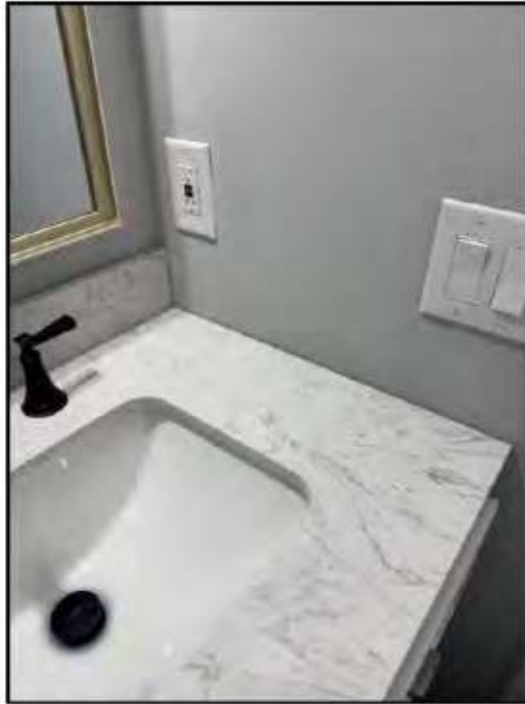
164. Caulking loose, missing or deteriorating
