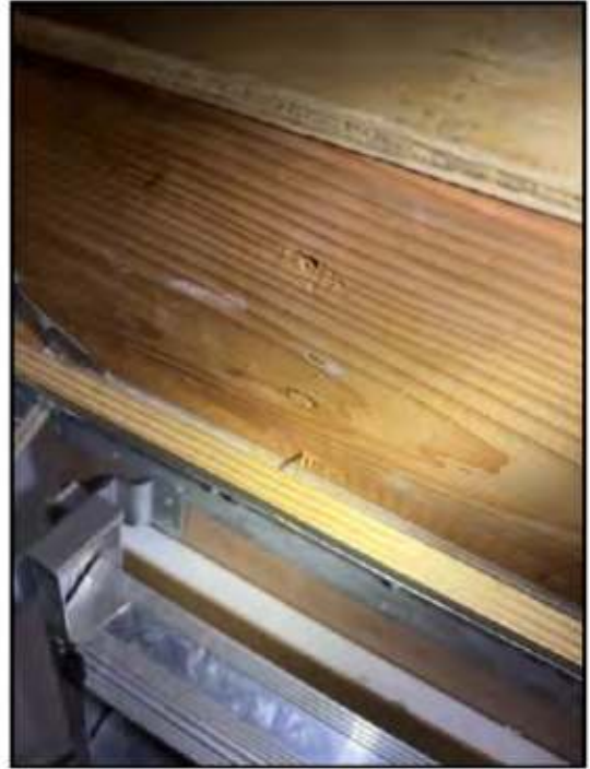
150. Not well secured
