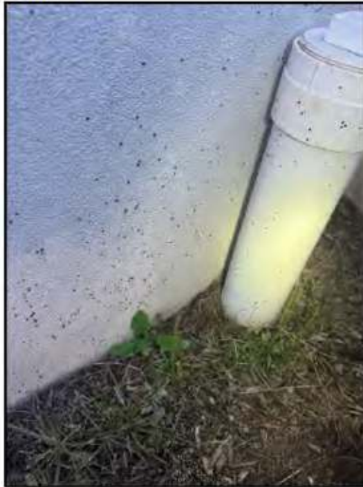
87. Possible water infiltration behind EIFS
