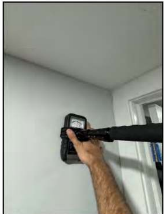
184. Active water leak detected
