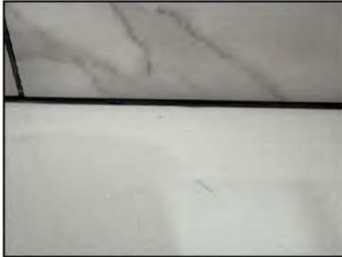
215. Caulking cracked or deteriorating
