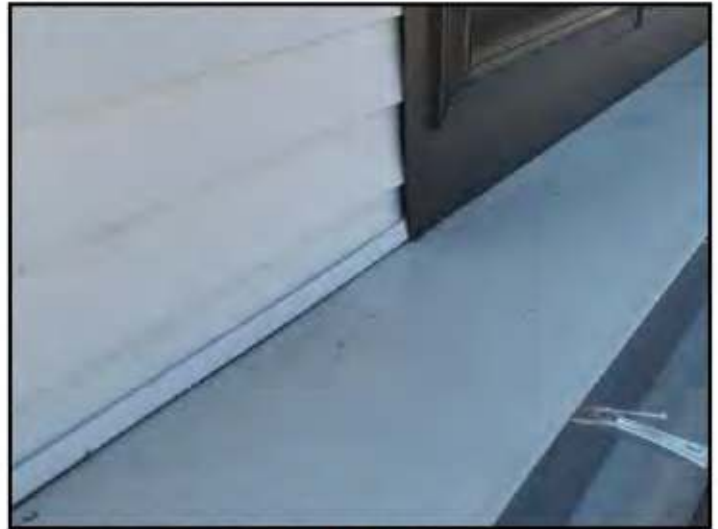
4. Possible water infiltration behind EIFS
