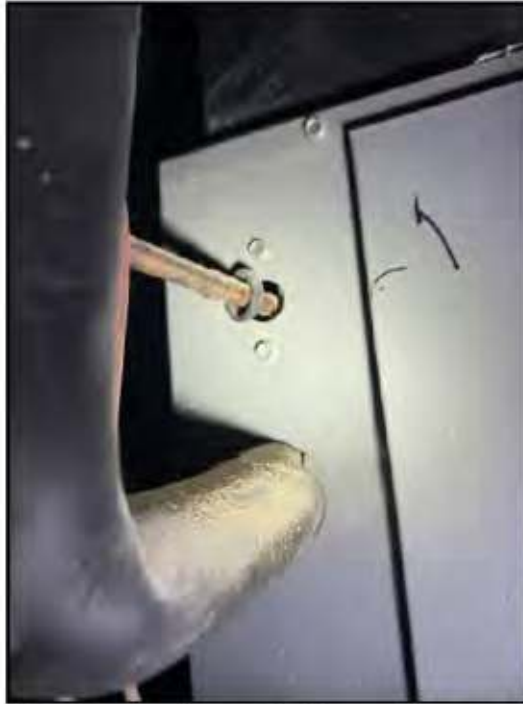
145. Poor seal around refrigerant lines entering...
