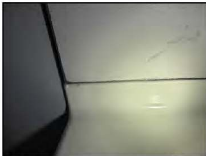
165. Bathtub weep holes were covered/clogged wit...
