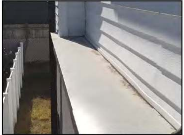
2. Possible water infiltration behind EIFS
