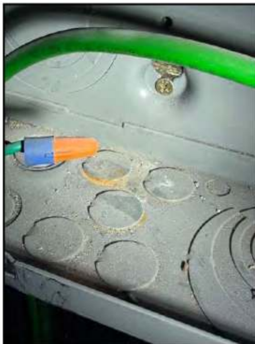
115. Rust or water in panel
