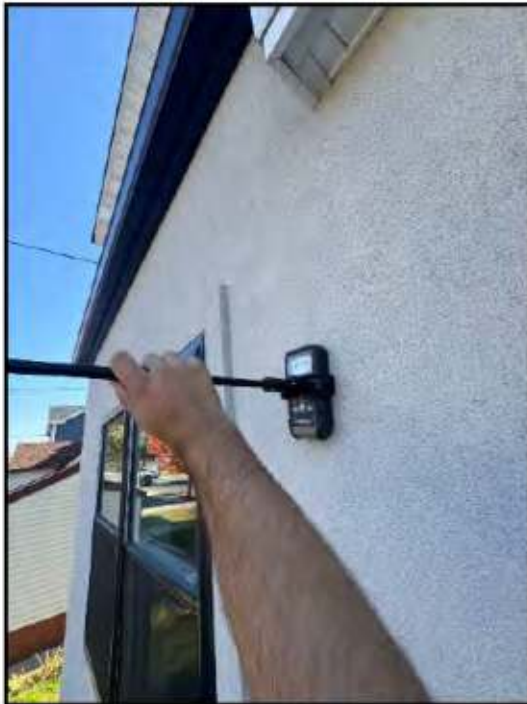
83. Possible water infiltration behind EIFS
