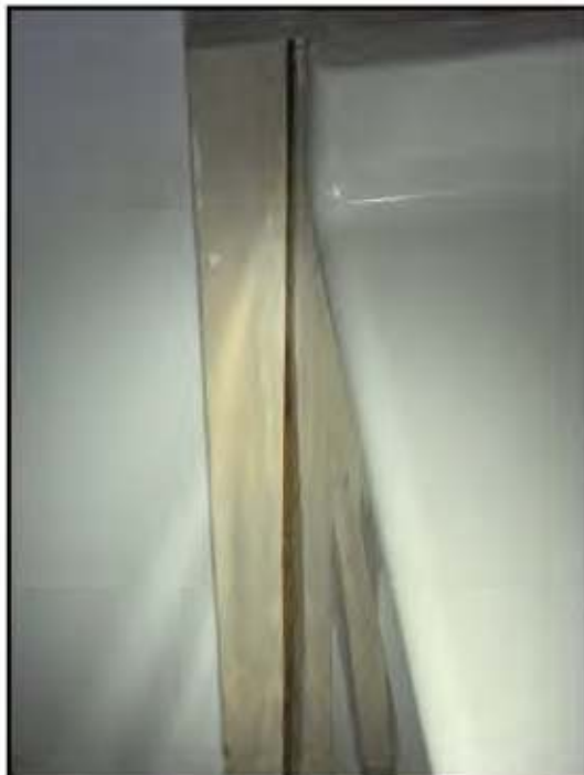
169. Tile loose, broken or missing
