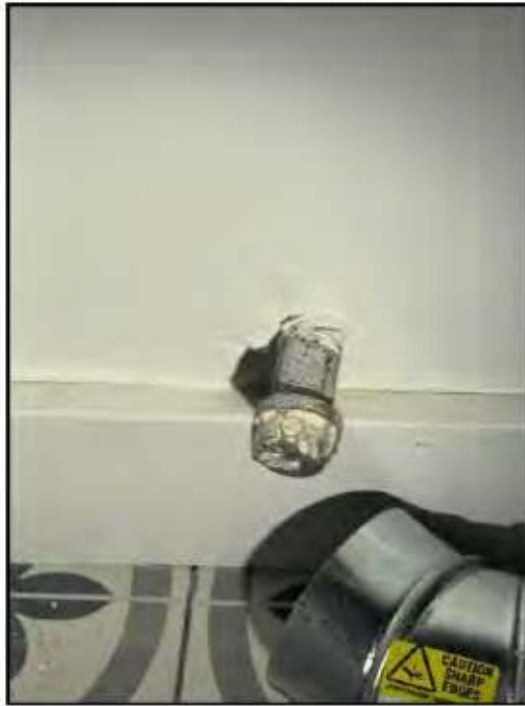
152. Missing shut off valve
