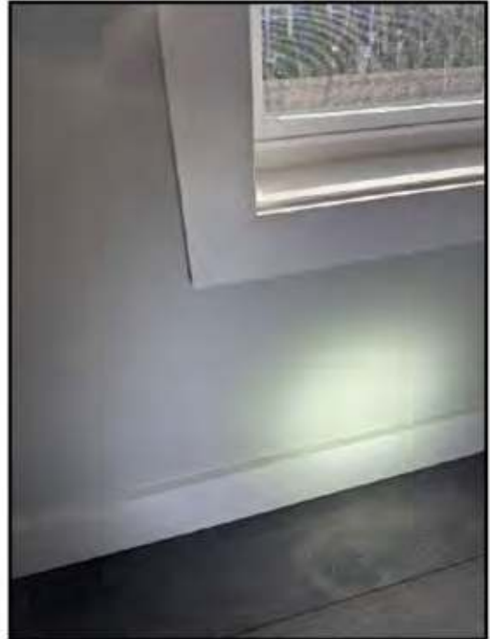
182. Active water leak detected
