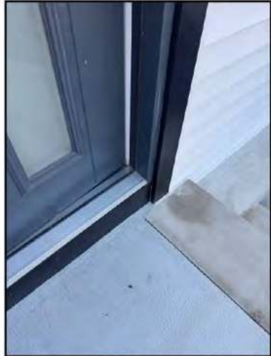
95. Damaged, cracked or loose
