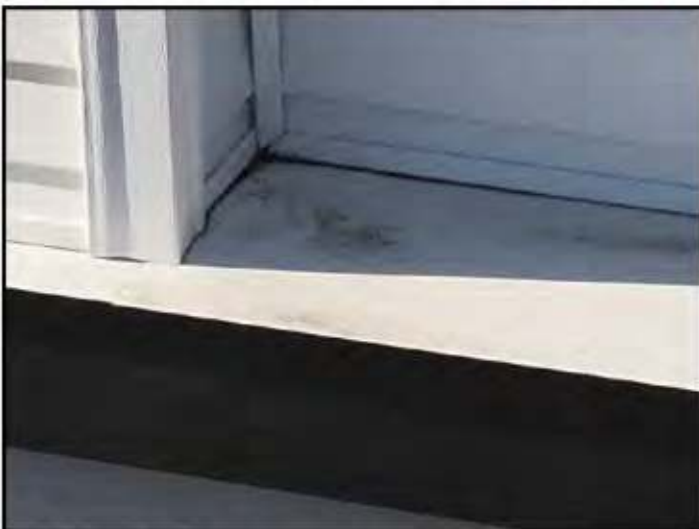
77. Possible water infiltration behind EIFS
