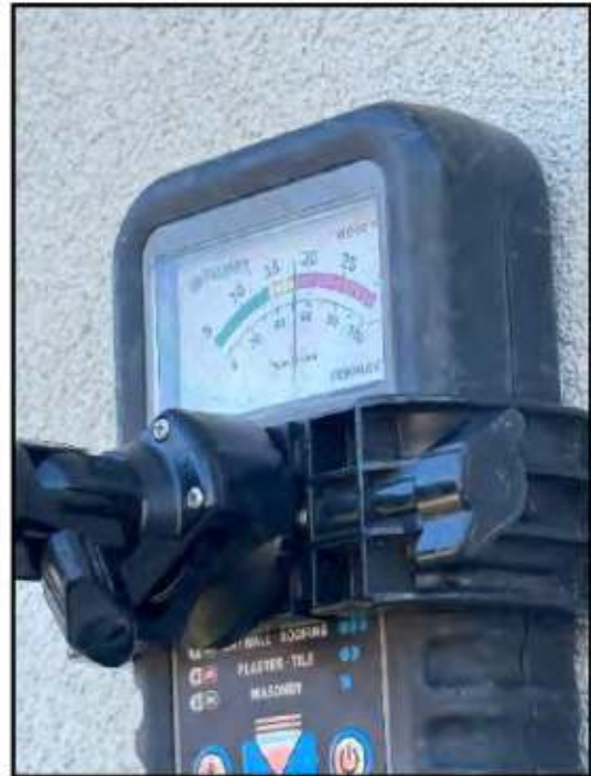
6. Possible water infiltration behind EIFS
