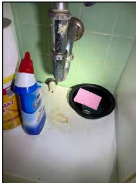
178. Possible leakage stains
