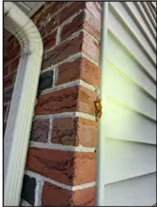
79. Openings between stone veneer and siding
