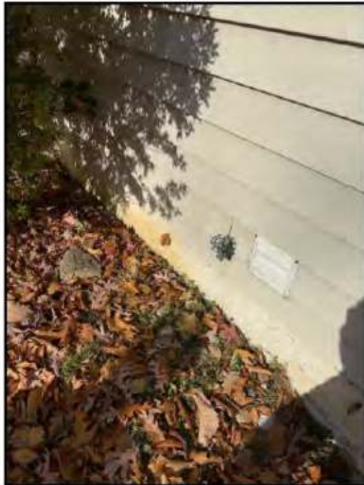
90. Improper slope or drainage
