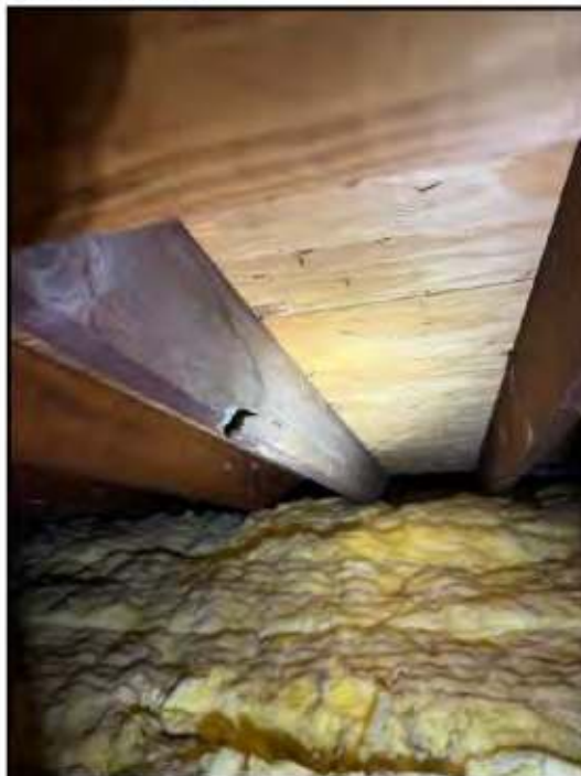
1. Split or damage
