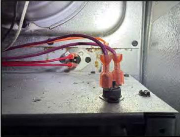
149. Rust, dirty, obstructed
