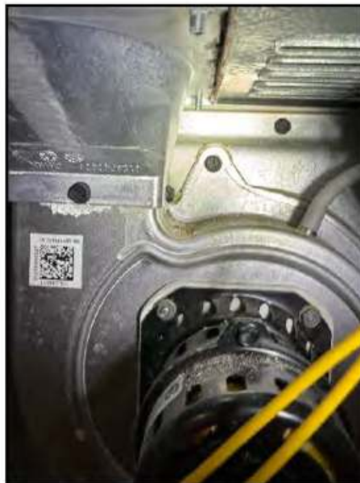
151. Rust, dirty, obstructed
