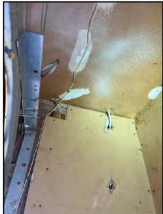
231. Missing sections of fire rated wall/ceiling...
