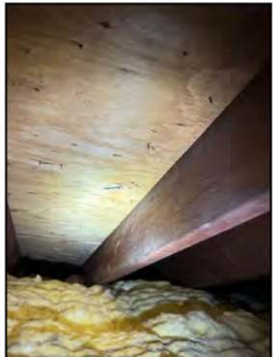
2. Split or damage
