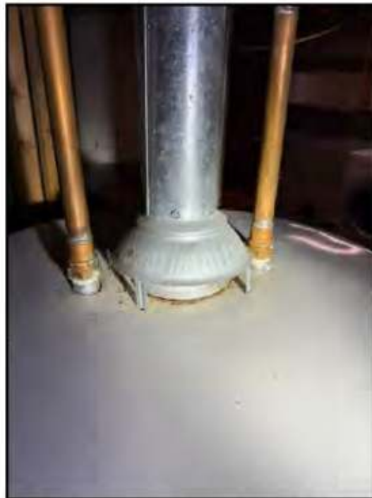
32. Vent connector too small, too big for water...
