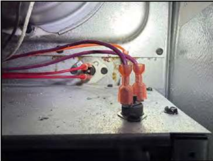
25. Rust, dirty, obstructed
