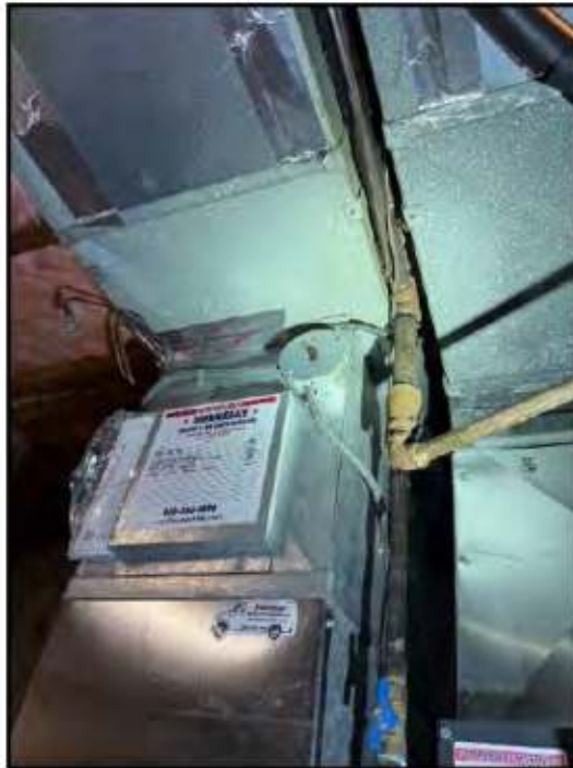
144. Furnace shut off switch must be marked with...
