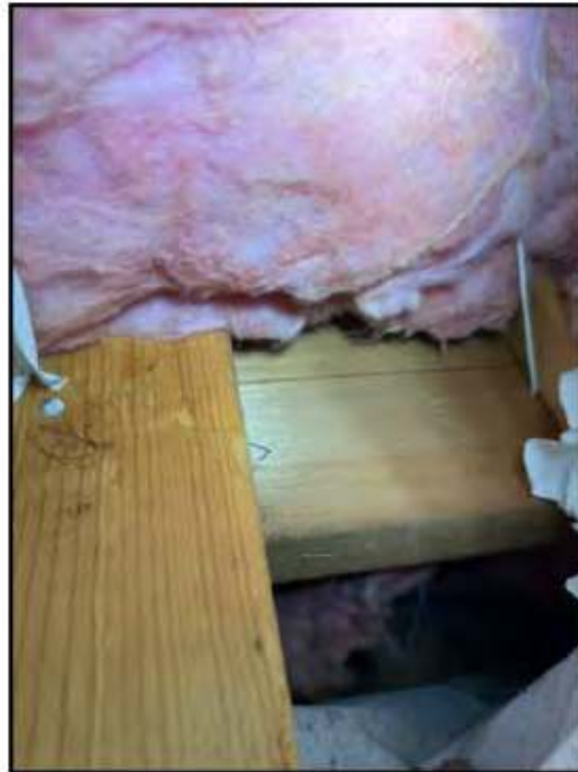
97. Split or damaged
