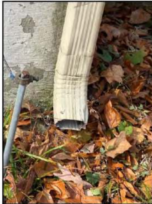
69. Discharge too close to building
