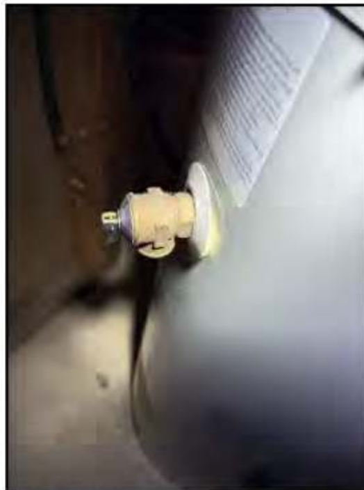
170. Discharge tube missing
