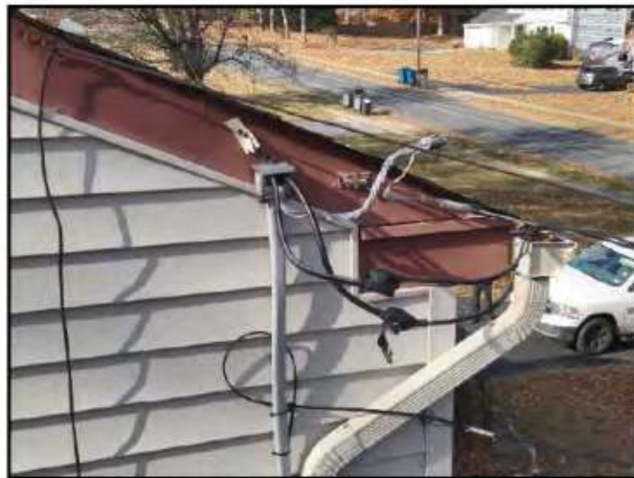
13. Poorly installed drip loop
