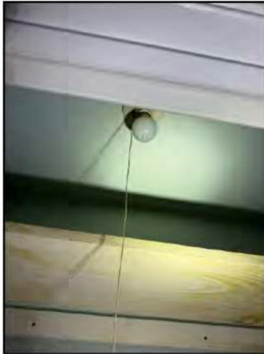
142. Too close to combustibles
