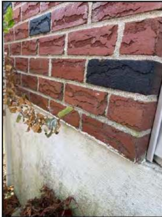
76. Missing, ineffective weep holes or flashings
