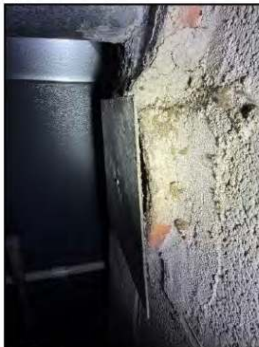
28. Abandoned openings for flue connections
