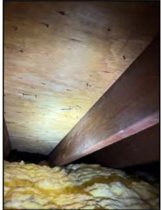
107. Split or damage
