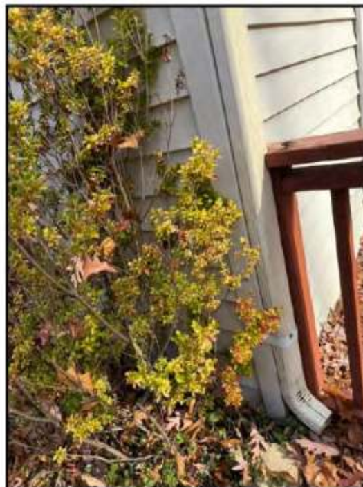
89. Trees or shrubs too close to building
