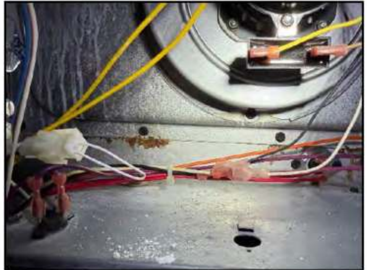
26. Rust, dirty, obstructed
