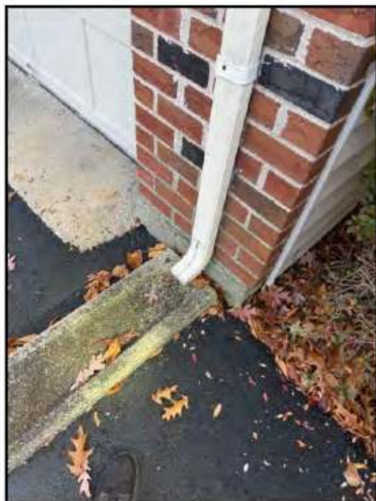
67. Discharge too close to building
