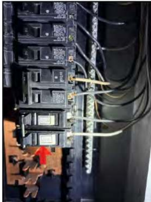
129. Older breakers in use
