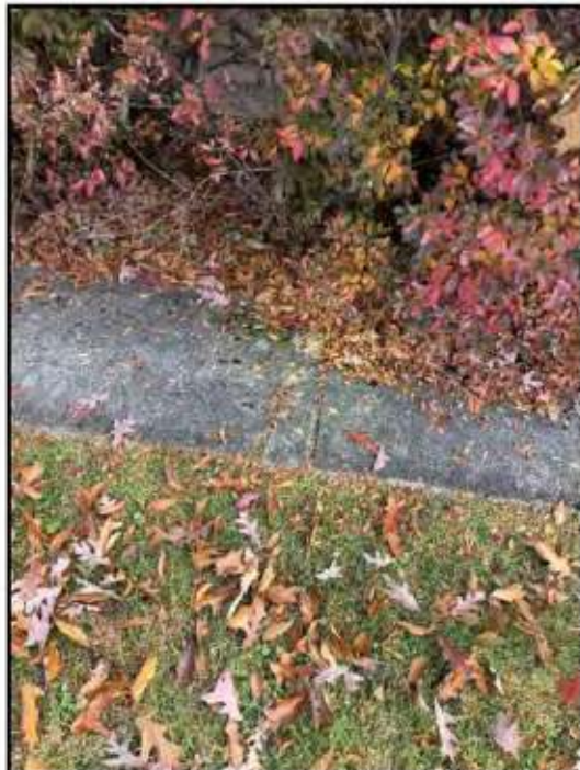
92. Cracked or damaged surfaces
