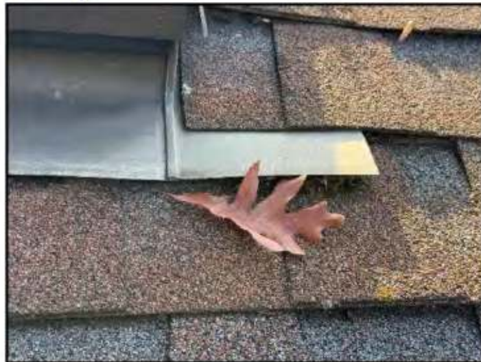
63. Open seams at flashings
