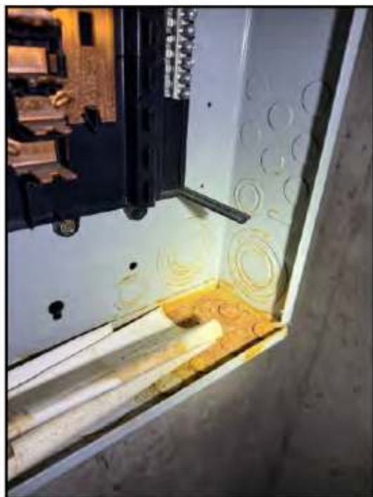
125. Rust or water in panel
