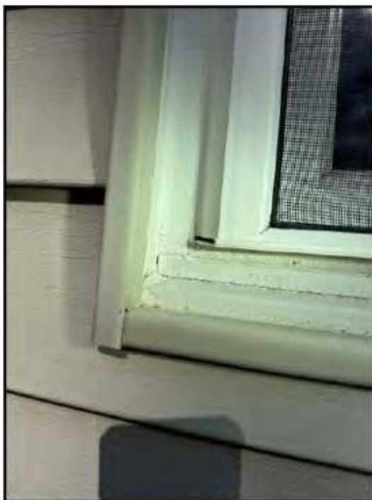
80. Caulking missing, loose or deteriorated
