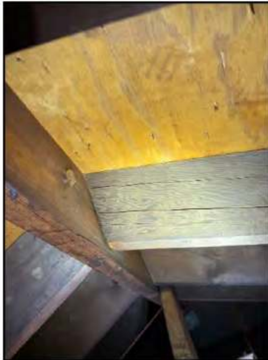
3. Split or damage
