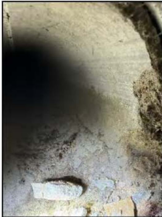
238. Possible asbestos containing materials
