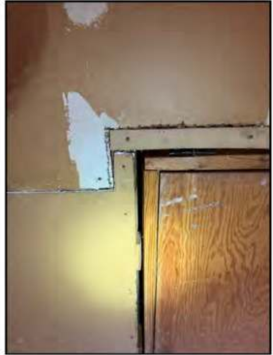
233. Missing sections of fire rated wall/ceiling...
