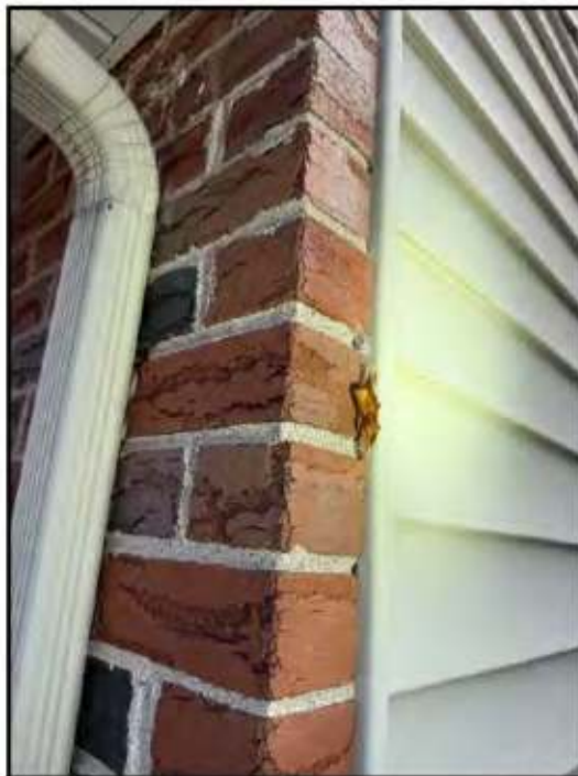
77. Loose brick veneer
