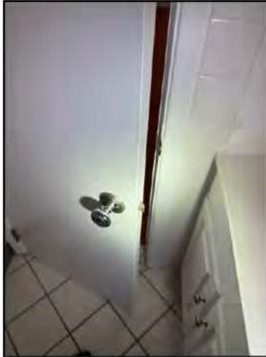
211. Does not latch properly
