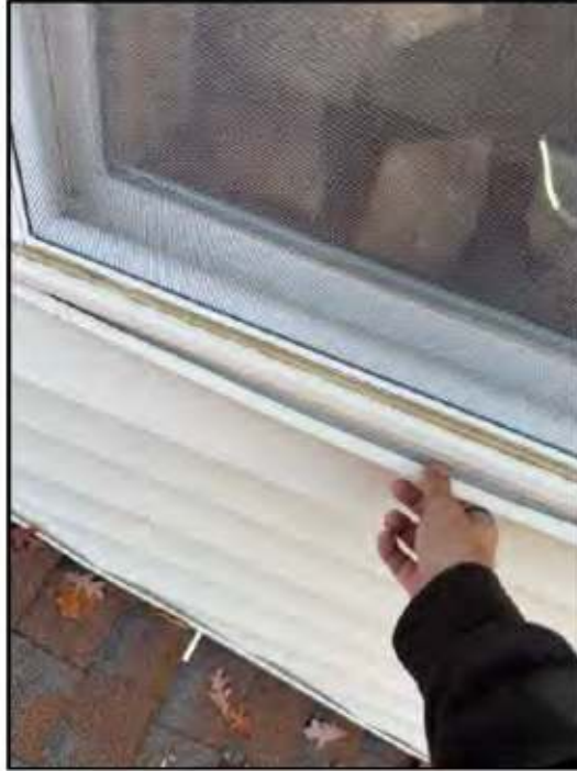
72. Loose or missing pieces
