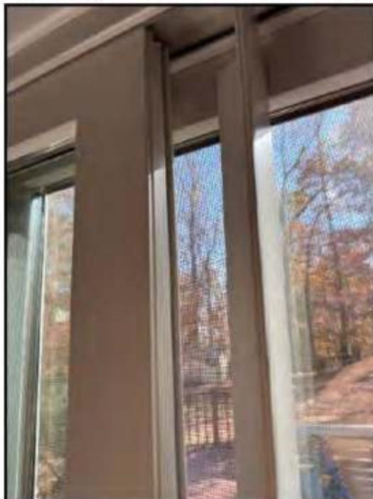
210. Weatherstripping missing or ineffective
