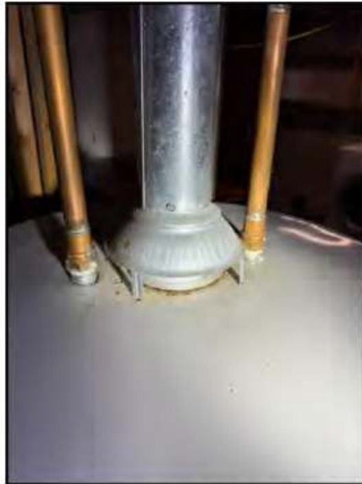
171. Vent connector too small, too big for water...
