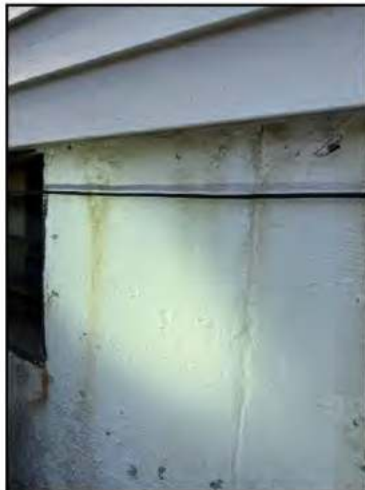
75. Possible signs of water intrusion behind...
