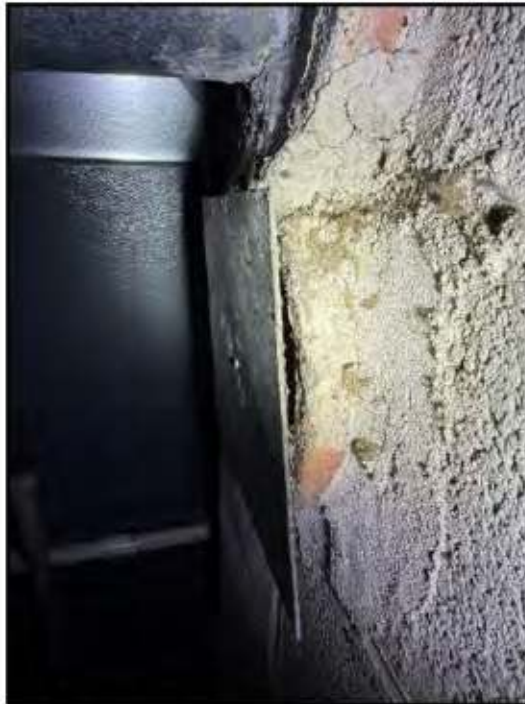
152. Abandoned openings for flue connections
