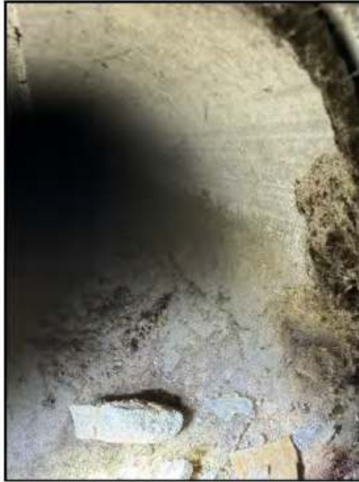
51. Possible asbestos containing materials
