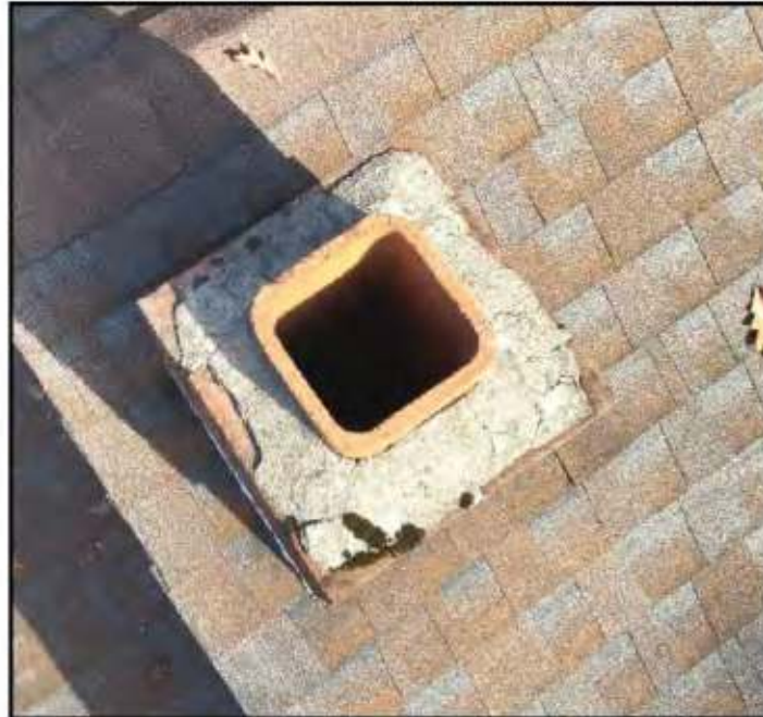
157. Rain cap missing or damaged
