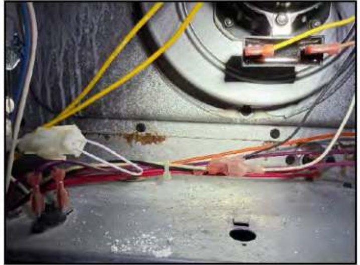
150. Rust, dirty, obstructed
