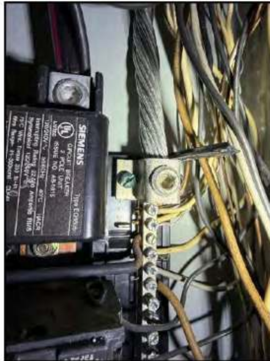
16. Rust or water in panel
