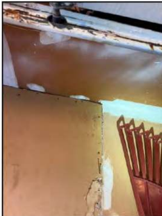
230. Missing sections of fire rated wall/ceiling...
