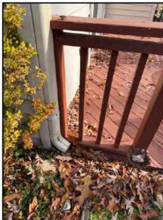
68. Discharge too close to building
