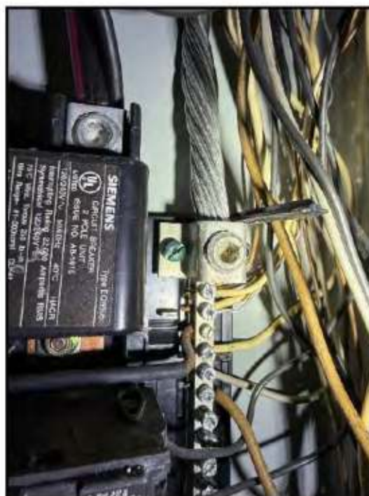
127. Rust or water in panel
