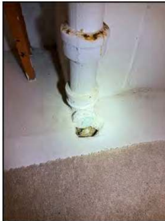
172. Clean-outs missing or inaccessible
