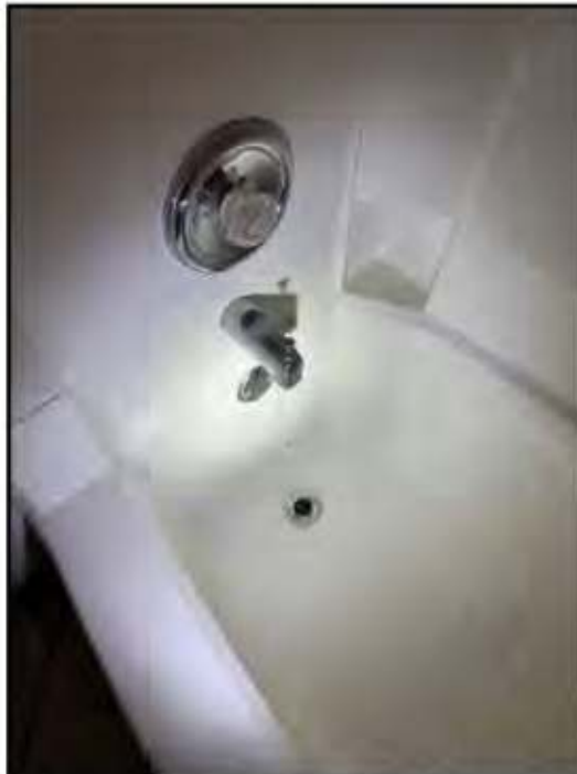
37. Loose shower valves/mixer piping
