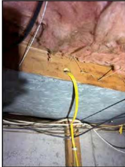
146. Return chase or plenum contain pipes, wires...
