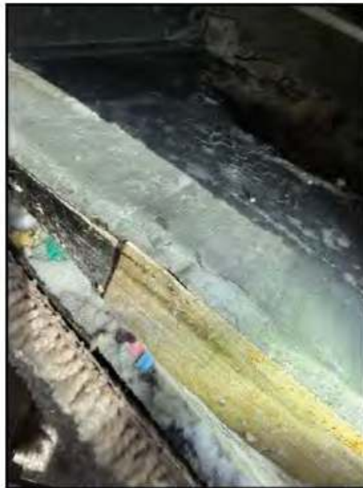
50. Possible asbestos containing materials
