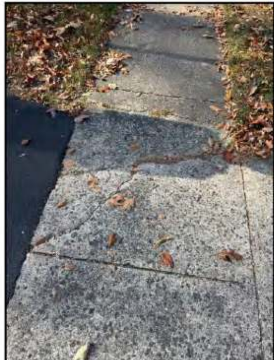
93. Cracked or damaged surfaces
