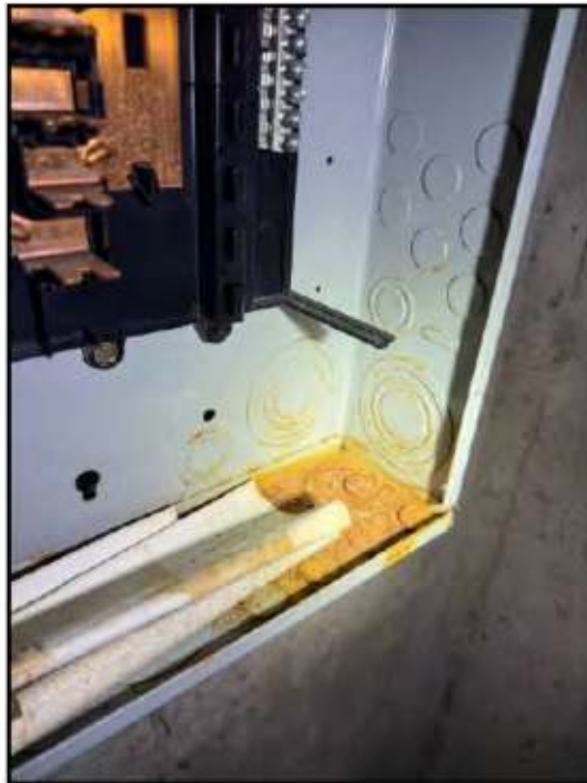
14. Rust or water in panel
