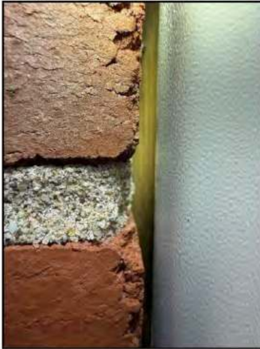
78. Openings between stone veneer and siding
