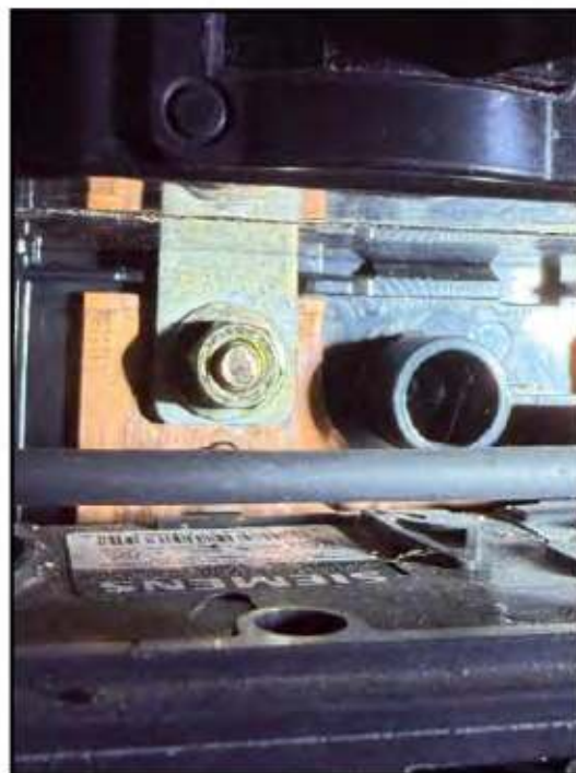
126. Rust or water in panel
