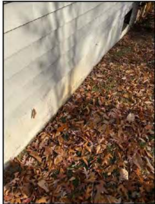
91. Improper slope or drainage
