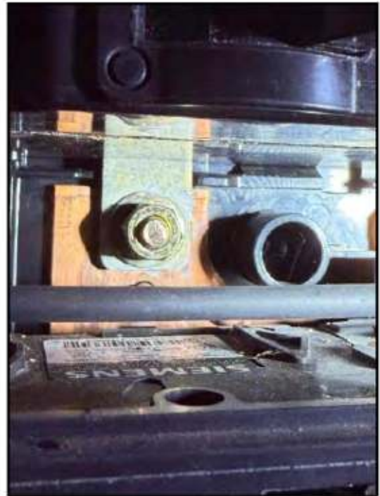
15. Rust or water in panel
