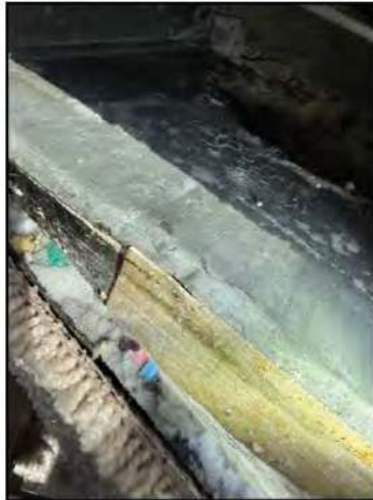
237. Possible asbestos containing materials
