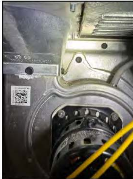
27. Rust, dirty, obstructed
