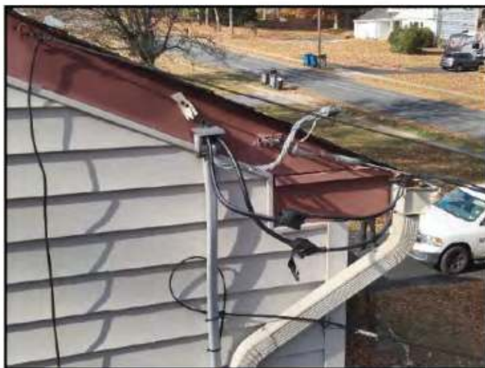
124. Poorly installed drip loop
