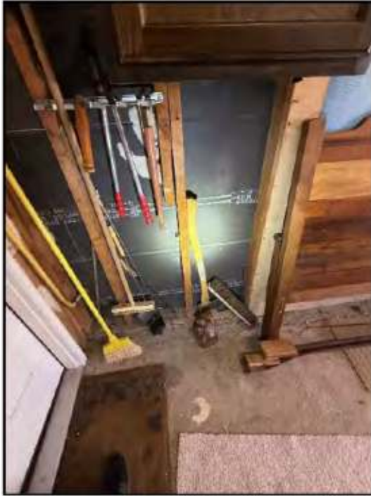
232. Missing sections of fire rated wall/ceiling...
