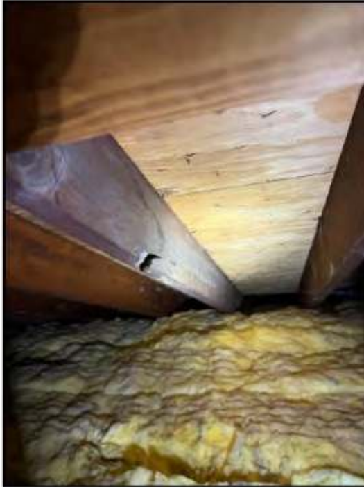
106. Split or damage
