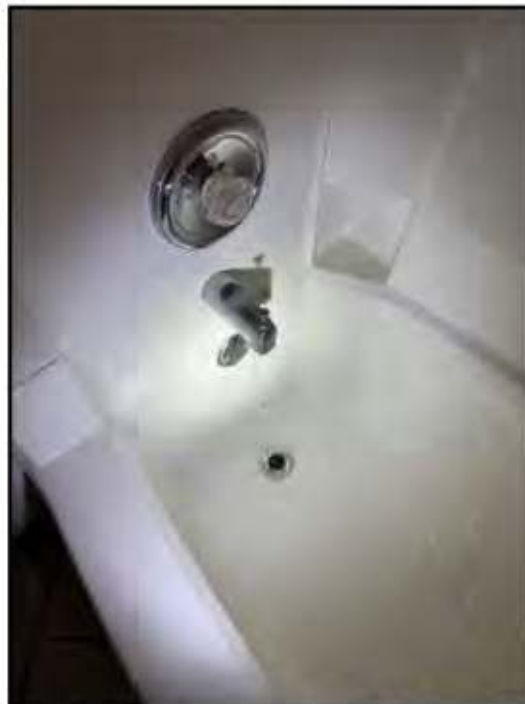
187. Loose shower valves/mixer piping
