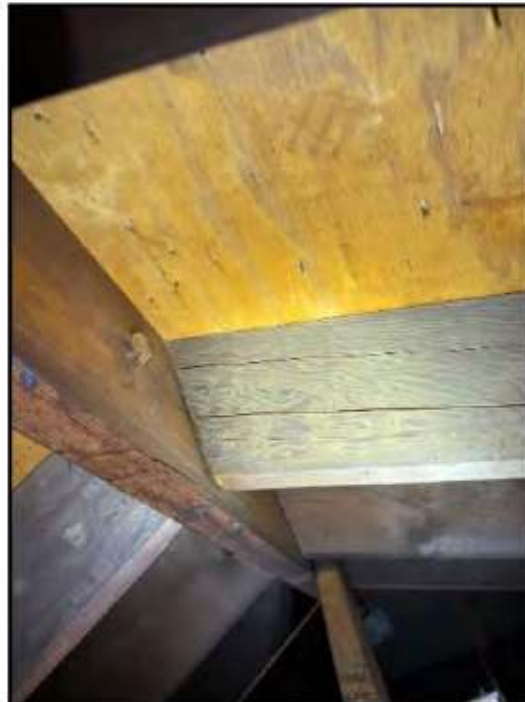
108. Split or damage
